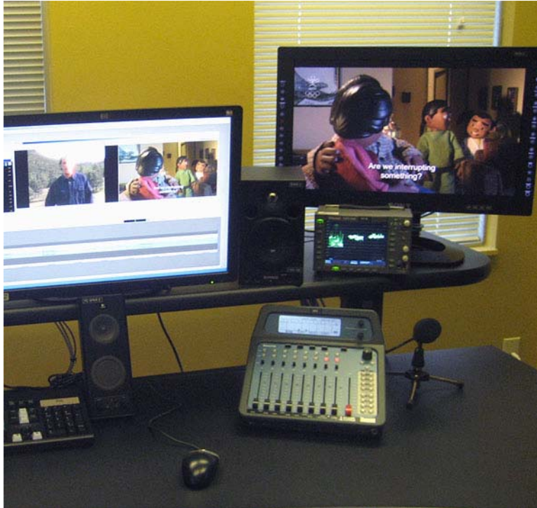
Renegade Labs Blue|328 Digital Mixer installed at APTN's Edmonton News Bureau
